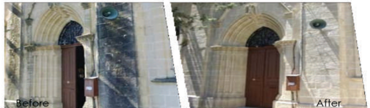
DeSalin C was used to remove algal greening and restore the surfaces of chapel in Dora, Cyprus. The porous walls were subsequently protected with SurfaPore C.
